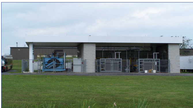
CATA's natural gas compressors.
